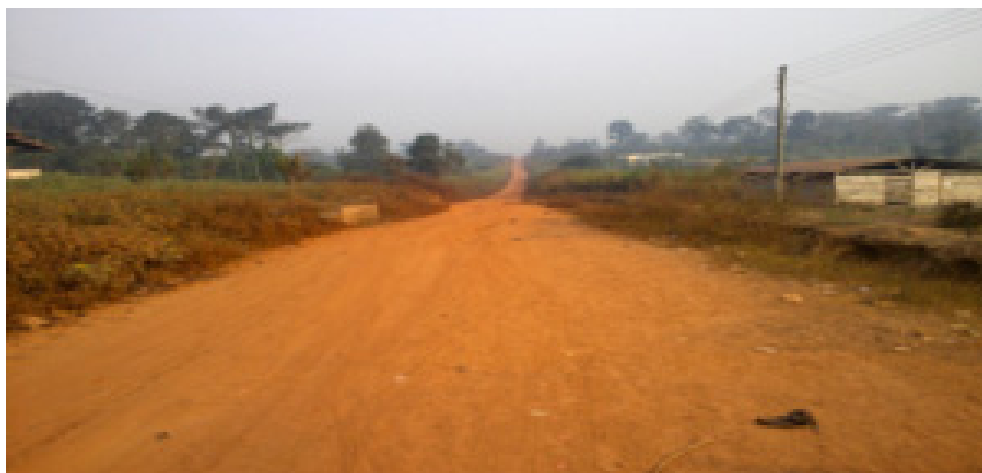
Photo 1 - Third class (graded earth) road linking one of the Communities to the main highway. Source: Author (2011)
